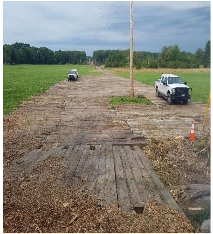
Fig 22: Timber matting installation through Frink Farm. Viewing west from Nimble Hill Road. (8-21-19).
