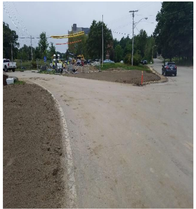
Fig 12: Restoration along Colovos Road and the road to Gregg Hall. Viewing south. (8-17-19).
